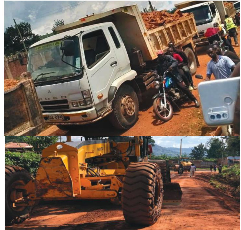
Maintenance of the roads ongoing Igare-Materio-Borangi, Nyamache-Mogonga, Mogonga-Emenwa, Riamamwana-Riamarube-Nyambunde, Nyamokenye-Kenyerere and Rise-Nyambunde. Photo | courtesy.
