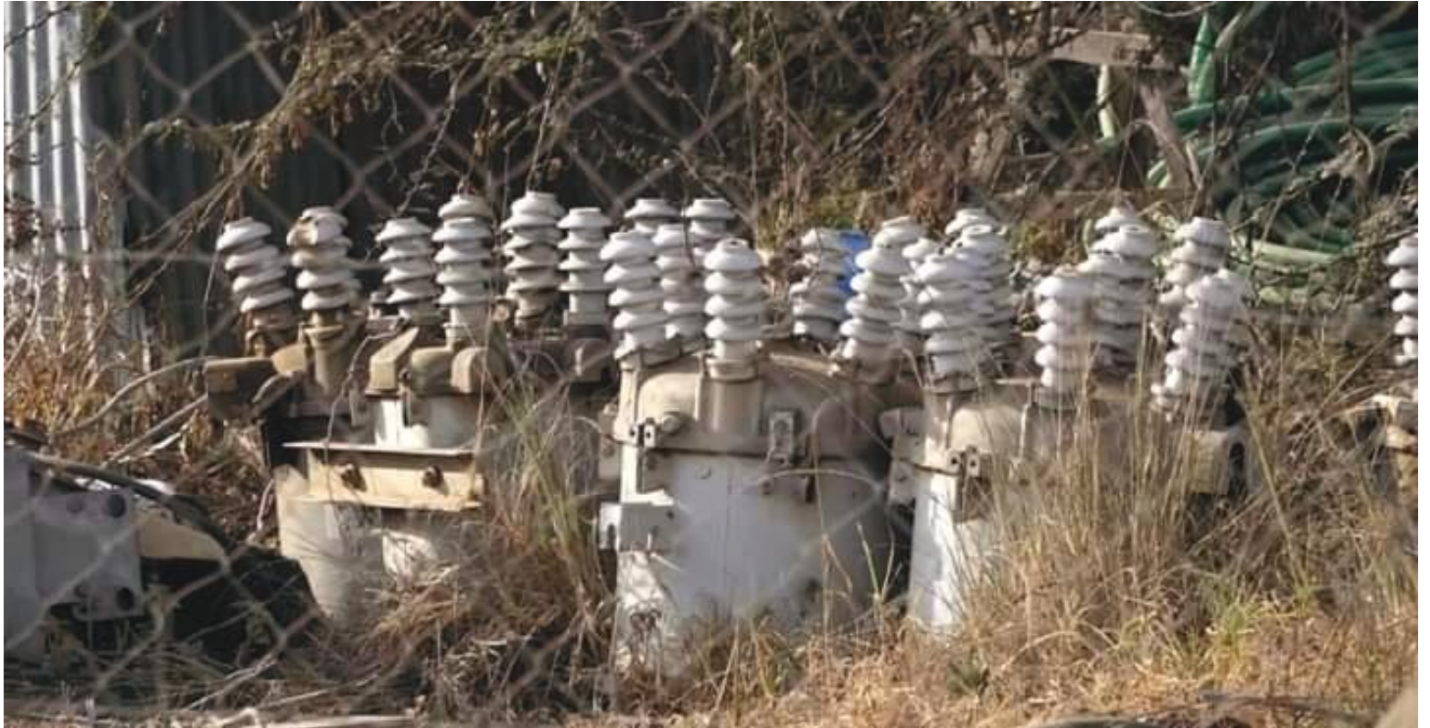
andalism Of Critical Infrastructure
