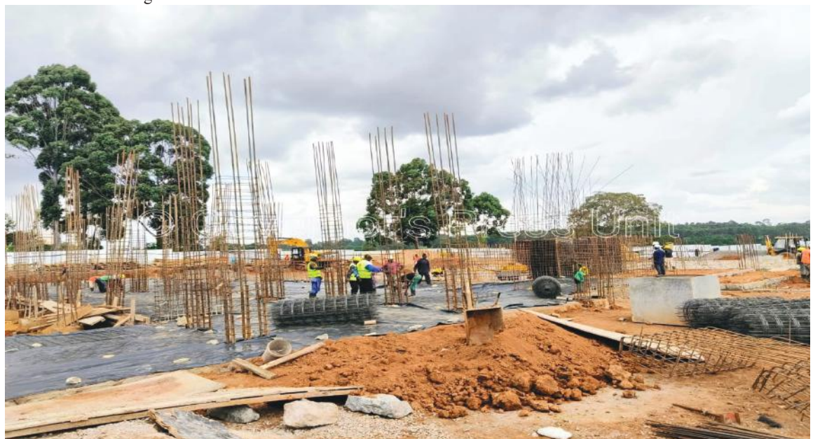
The construction of the state-of-the-art County's new Headquarters and Mother Baby Unit in Tom Mboya Health Facility are currently ongoing.
