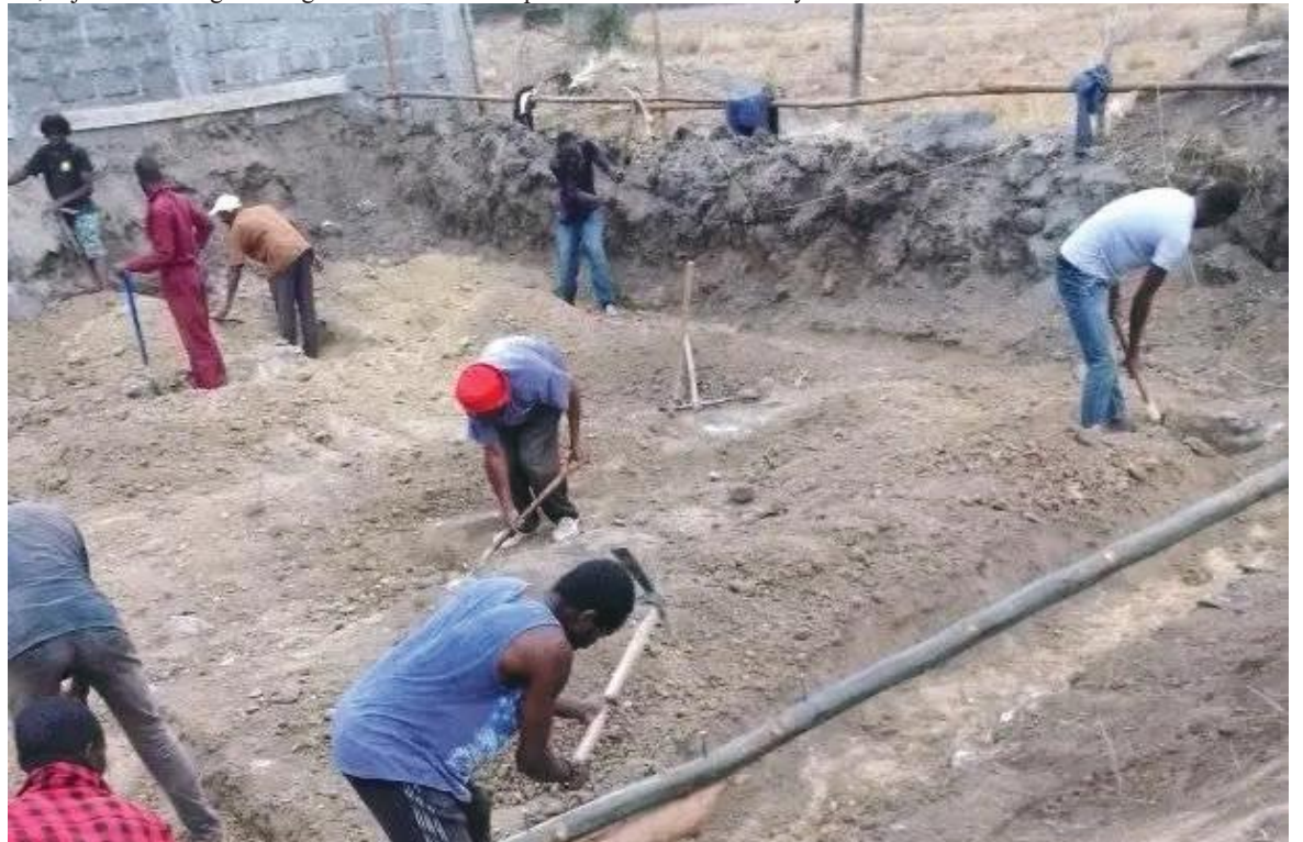
People working in a construction site without protective gear .
