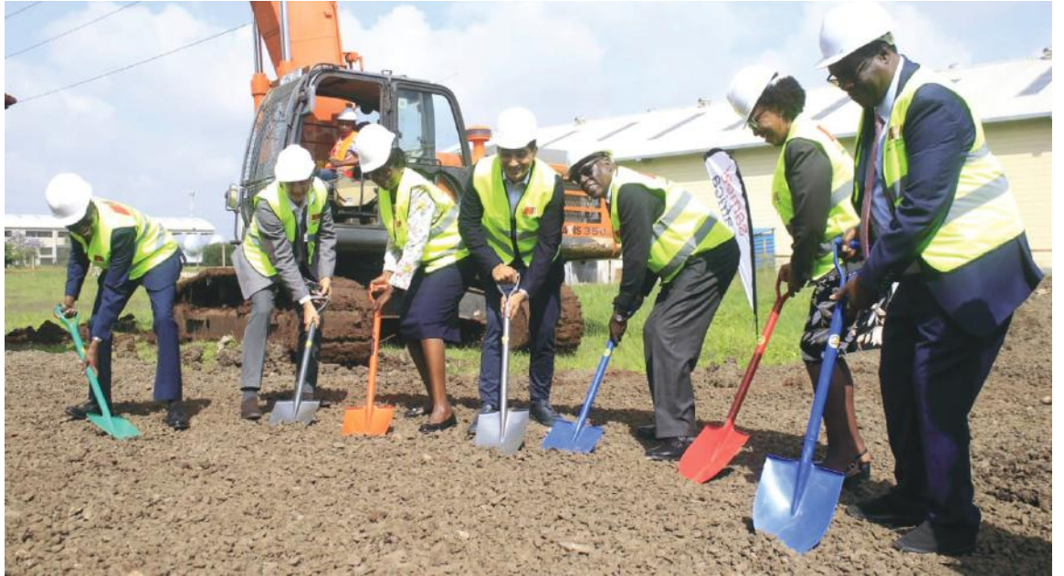
Left to Right) Sameer Africa MD John Mugo accompanied by Sameer Africa board members Akif Butt, Mary Ngatia, Sameer Mer-ali, Eng. Erastus Mwangera, Dr. Lydia Mbuthia and Peter Gitonga during the ground breaking of Sameer Africa Ksh 260 Million Purpose-Built Industrial Warehouse.
