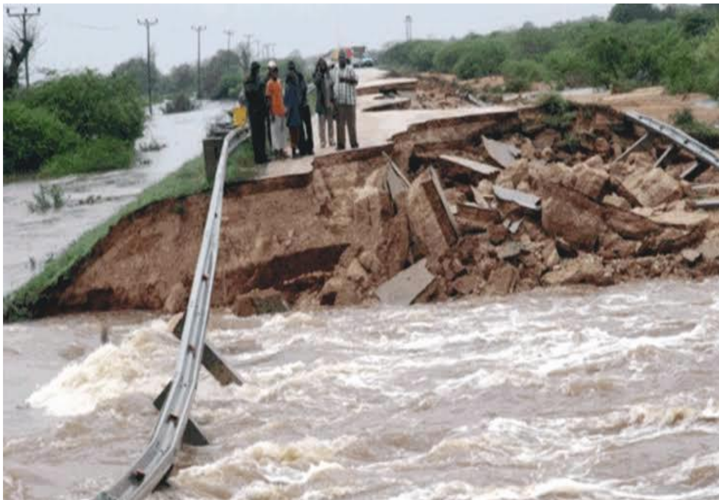
Bridge Affected By Heavy Floods.
