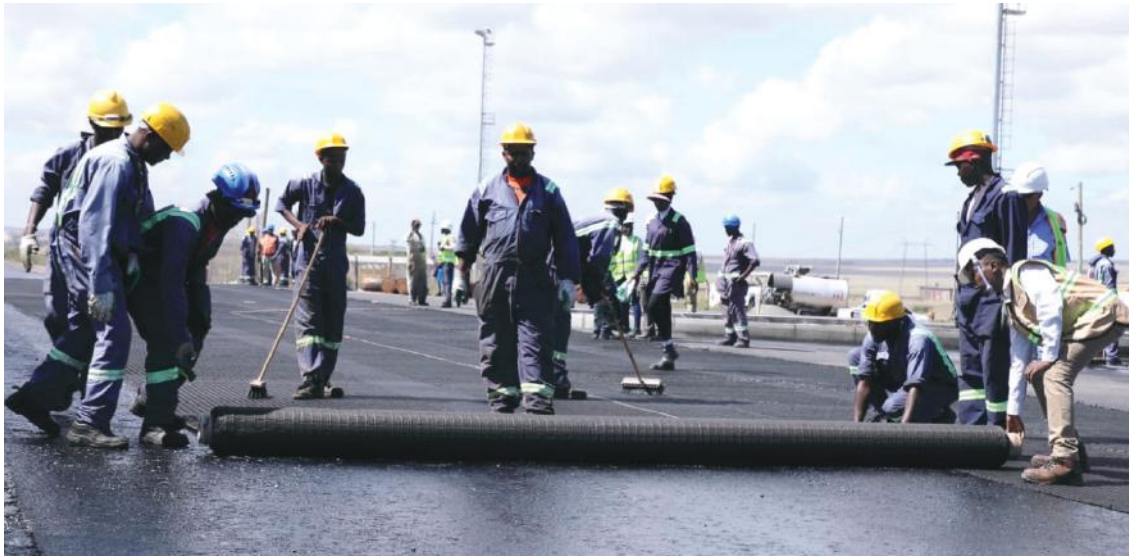
Admir Technologies Kenya Country Manager Eng. Anthony Irungu (right) guides road construction technicians applying Asphalt reinforcement grids at Konza Technopolis
