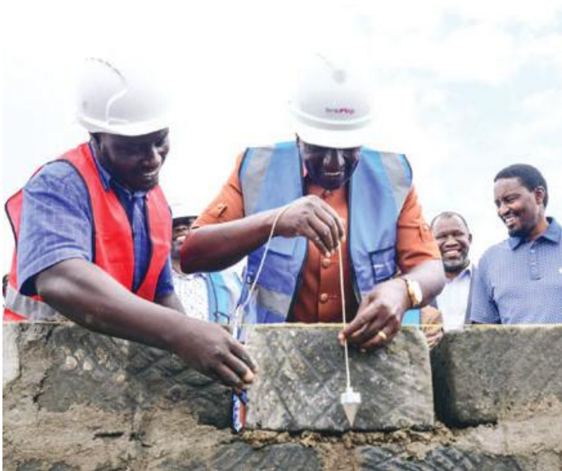
Jan 10, 2024 | President William Ruto lays a stone while commissioning an affordable housing project in Laikipia/PCS
