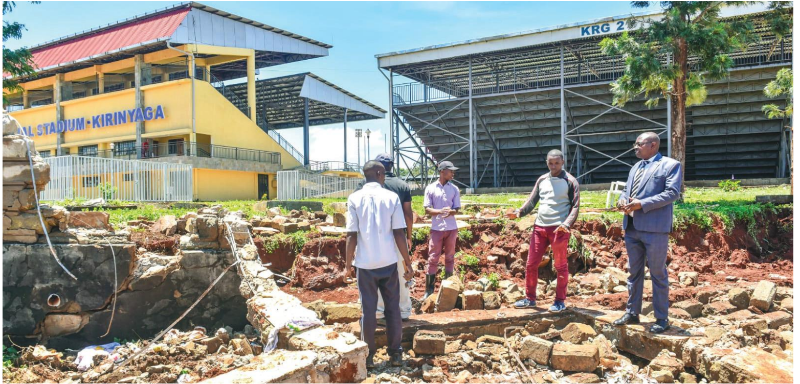
Kirinyaga CECM for Roads, Transport and Public Works, Jared Migwi, assessing a section of Wang'uru Stadium perimeter wall that was destroyed by heavy rains.
