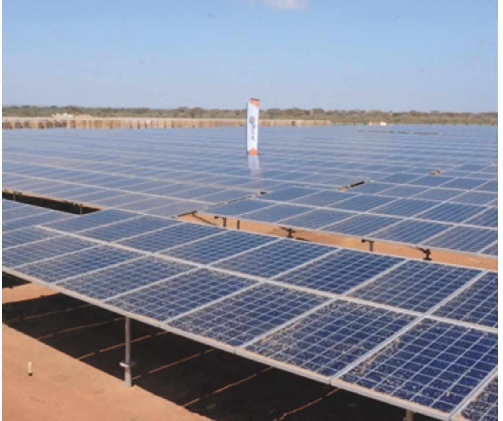
Located in northeastern Kenya, the Garissa Solar Power Plant is the first major solar plant to tap into the country's vast solar resources and the largest grid-connected solar power plant in East and Central Africa. /REREC.
