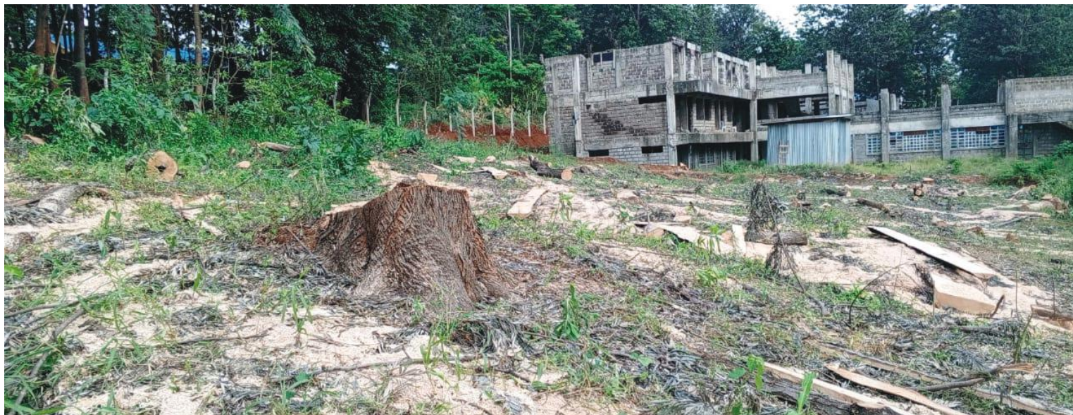
Photos showing cut trees at Kenya Medical Training College, Chuka campus construction site in Tharaka Nithi County.
