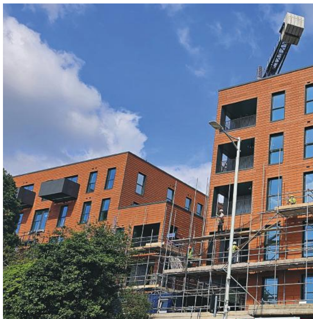
Desperately needed new homes under construction in London. At least 300,000 new houses are needed. Photo SHAMLAL PURI
