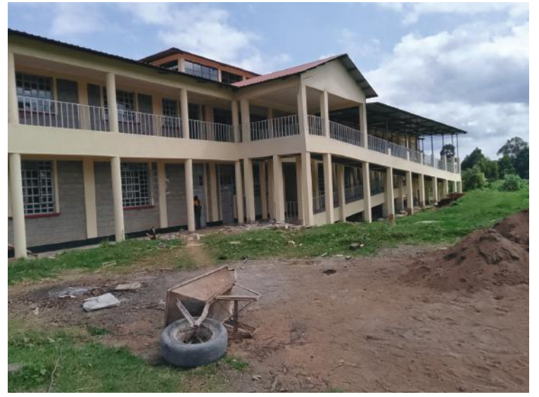
Gichugu Technical and Vocational College at Kiambatha village, Gichugu constituency, Kirinyaga County. PHOTO BY RAYMOND WANJOHI.
