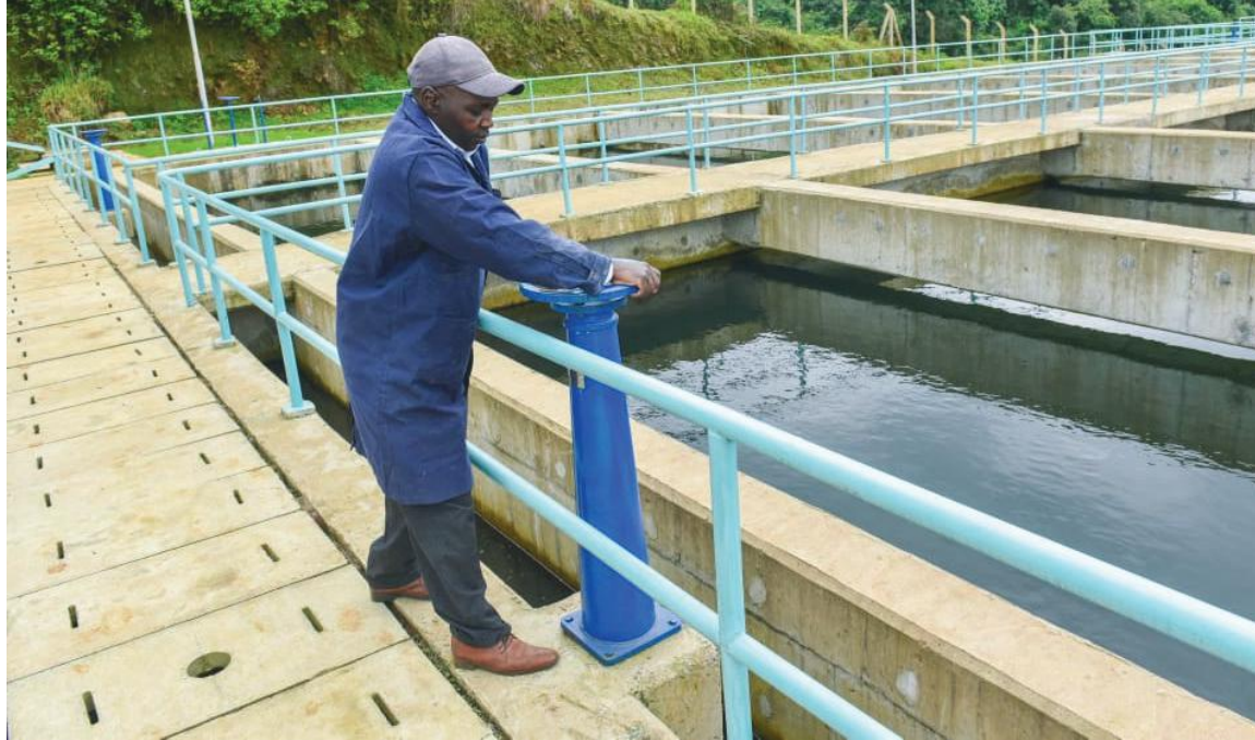
A technician test running the water systems..
