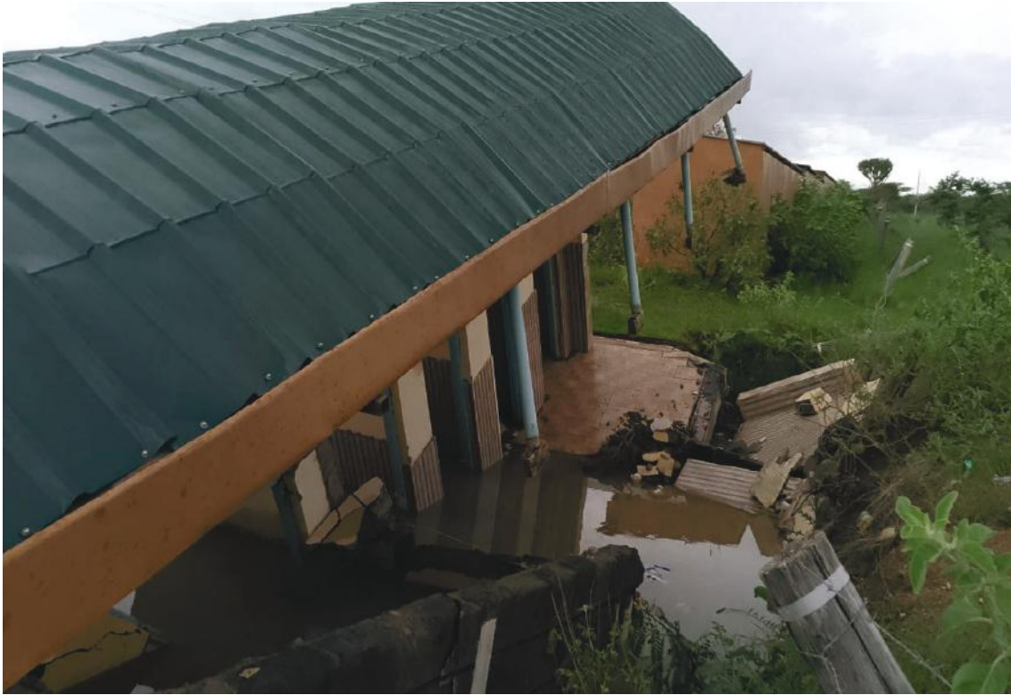
Part of Naibor market that is yet to be occupied falling apart. Photo/PAUL WANJIRU.
