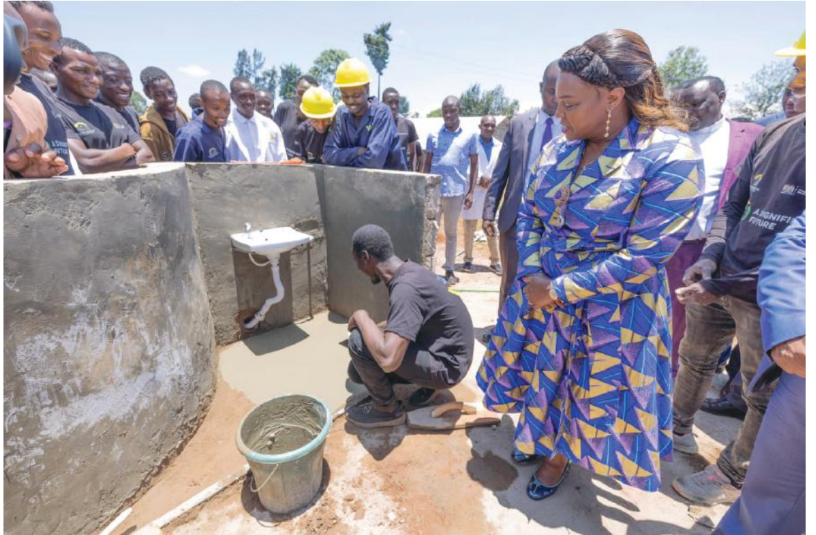
Pastor Dorcas Rigathi, the spouse of the DP watches as one of the beneficiaries of the boy child program in Ngorano, Nyeri County on Friday done finishing touches on a construction project during a day set aside to showcase skills gained by 303 men in plumbing, security, welding, fashion and design, and electrical installations.. Photo/ODP.
