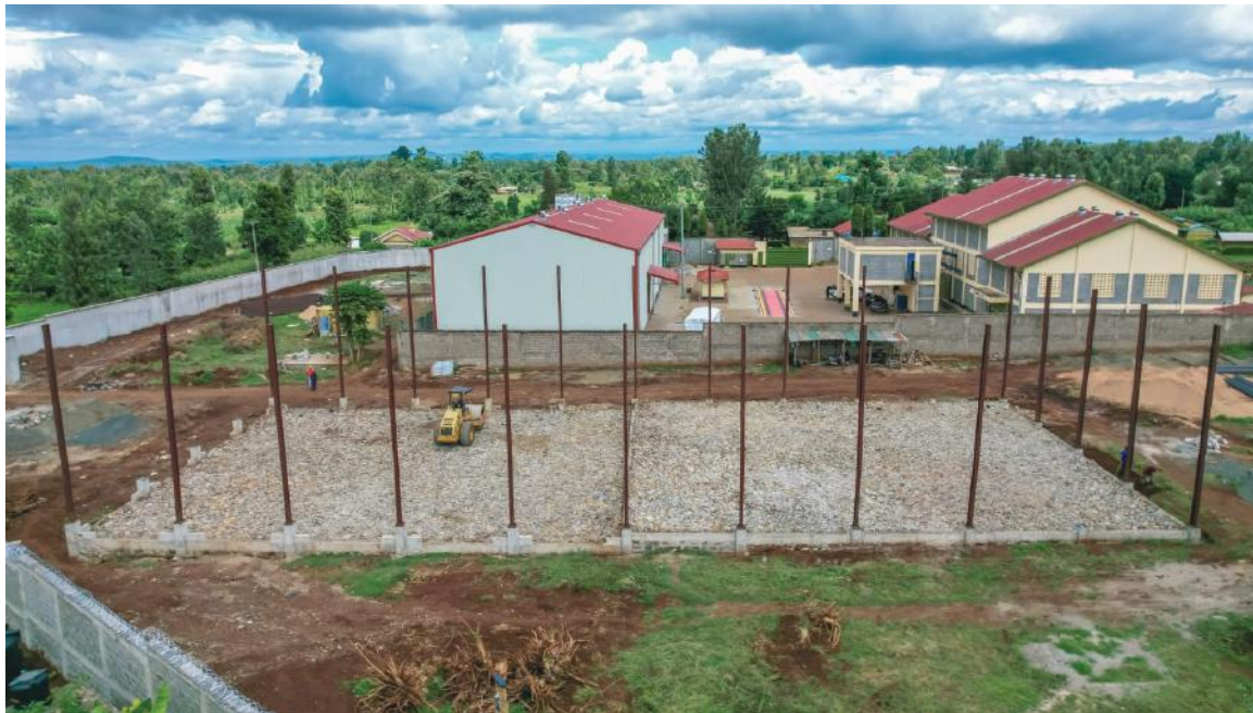
Ongoing Construction of a state of art Coffee Warehouse by Kirinyaga County Government that it set to transform Kirinyaga Cooperative Union operations.
