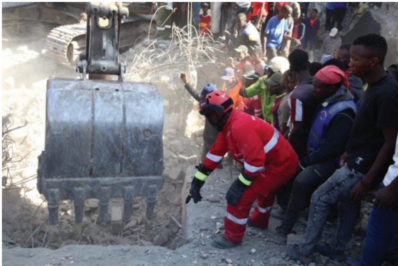
Shauri Moyo building collapse.
