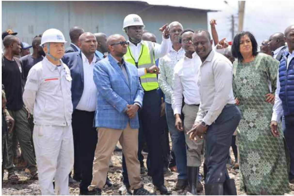
Nairobi Governor Johnson Sakaja with senior officials, including Woman Representative Esther Passaris, when he broke ground for the construction of the Gikomba modern market yesterday
