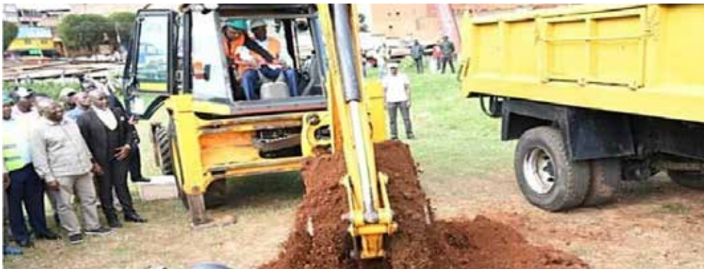
Deputy President Kithure Kindiki launching the construction of Othaya stadium last year. Looking on are leaders led by Othaya MP Wambugu Wainaina (standing centre). | Photo: Courtesy.
