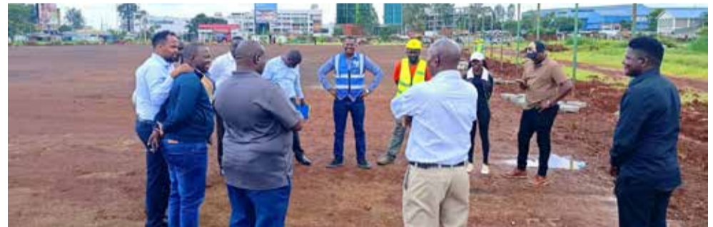
Ruiru Stadium upgrade, which officially began 12 days ago under Governor Kimani Wamatangi's administration in Kiambu County, is progressing steadily. A management team, led by County Youth Affairs, Sports, and Communication Executive (CECM), Osman Korar and Chief Officer for Sports, Godfrey Masolo, visited the site to inspect ongoing works. The contractor is currently constructing the drainage system and perimeter fencing. Upon completion of this phase, ground compaction will follow, paving the way for installation of a new astro-turf surface that will greatly enhance the pitch quality and usability.
