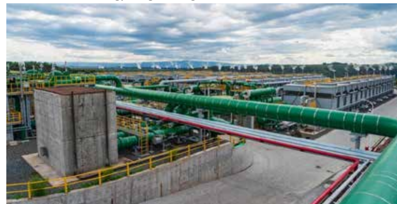
This photo taken on April 20, 2026 shows the Menengai Phase I Orpower 22 geothermal power plant project, constructed by China's Kaishan Group, in Nakuru County. | Photo: Xinhua/Xie Jianfei.
