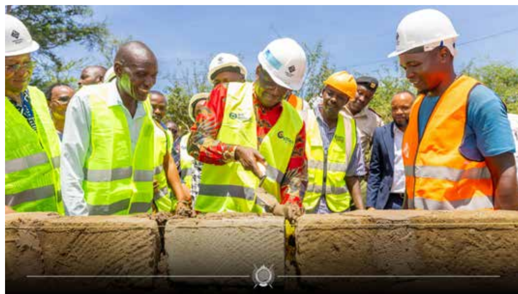
Tharaka Nithi Governor Muthomi Njuki laying foundation stone for CT scan building at Marimanti Level Four Hospital in Tharaka Constituency. | Photo: Alex Njeru
