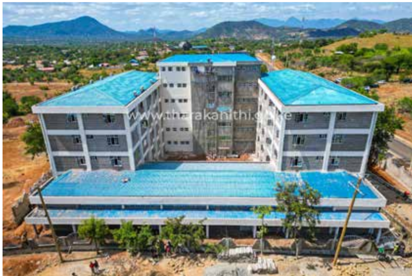
The near completion Tharaka Nithi County executive offices building at Kathwana. The building has been financed by the county government | Photo: Alex Njeru
