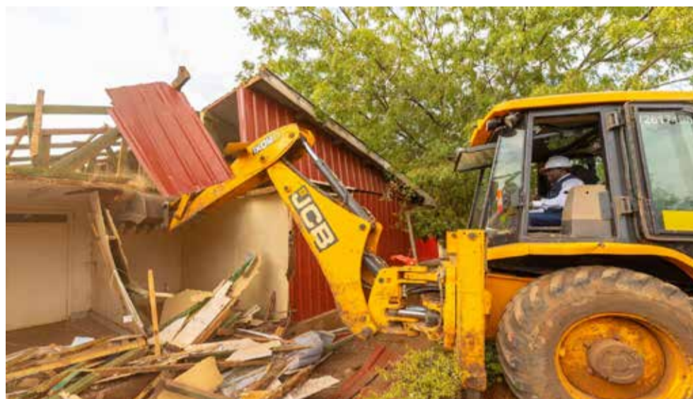
Tharaka Nithi Governor Muthomi Njuki during demolition of Kathwana county headquarters mabati offices that have been in use since 2013. | Photo: Alex Njeru.
