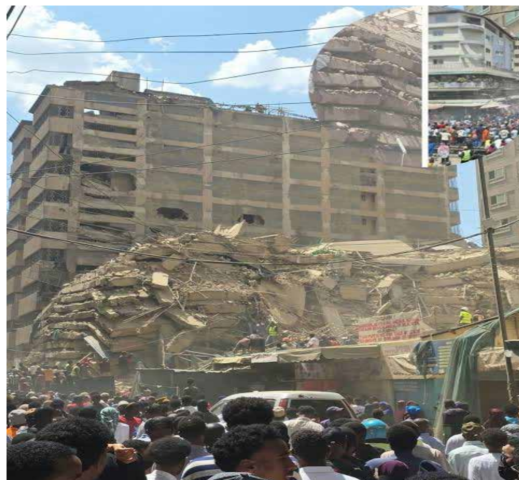
Collapsed multi-storey building on 9th Street in Eastleigh
